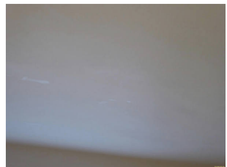
Overpaint marks RHS
