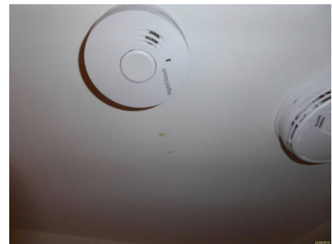
2 Alarms in hall
