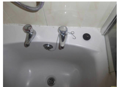
Mould marks behind bath taps
