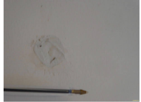
Repair mark LHS
