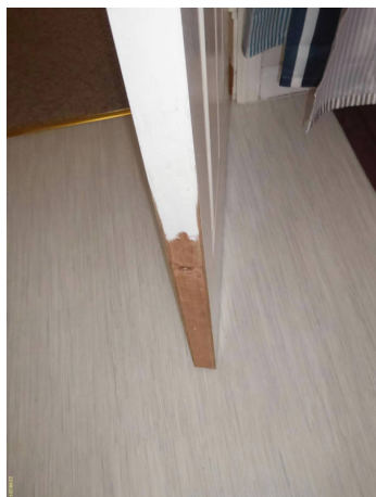
Leading edge of door rubbed down to wood
