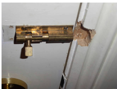
Reverse door lock catch plate missing
