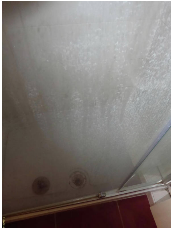
Shower cubicle limescale marked
