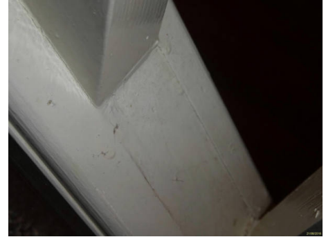
Dust on surfaces
