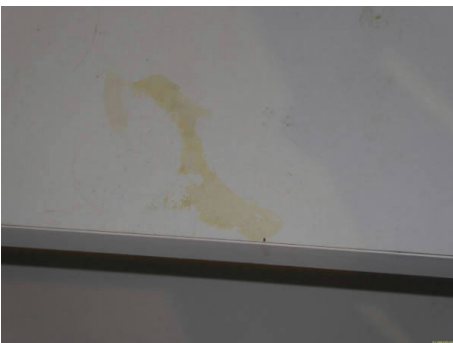
Units not clean
