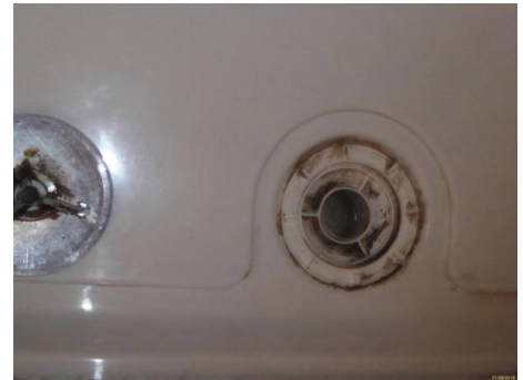
Shower wastes dirty
