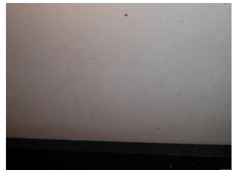
Grease marks above worktop
