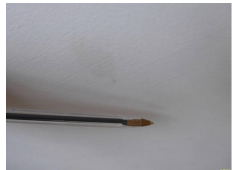
Scuffs on walls
