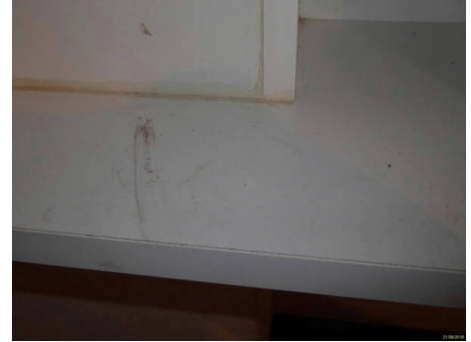
Units not clean
