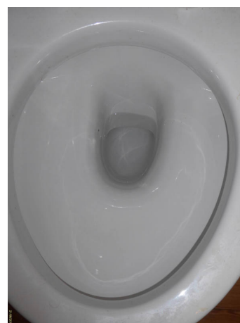
Stains top edge of toilet bowl
