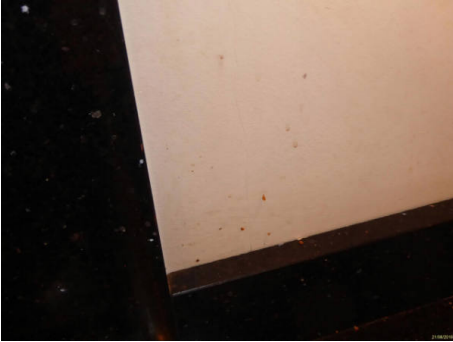
Grease marks above worktop
