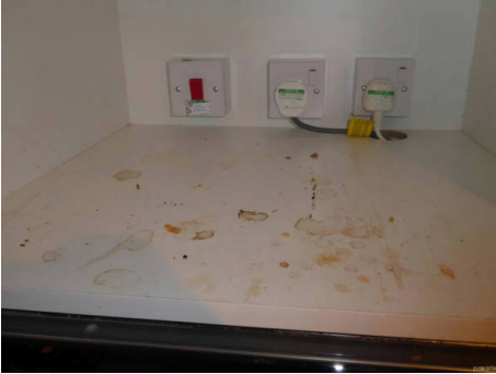
Units not clean
