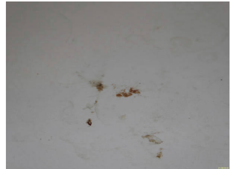
Units not clean
