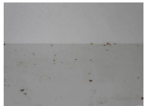
Units not clean
