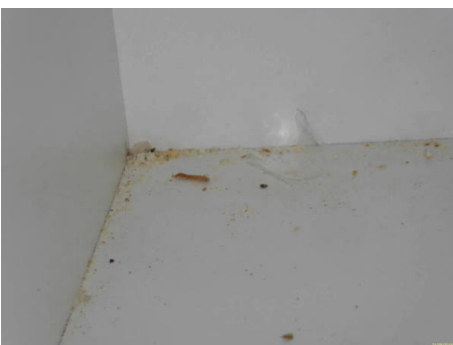
Units not clean
