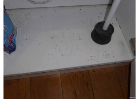
Units not clean
