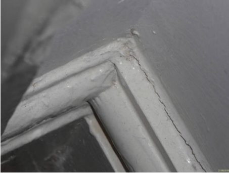
Skirting dusty on landing
