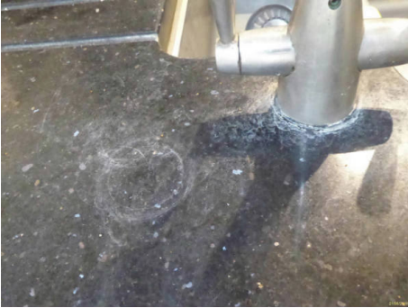
Limescale w/top base of taps
