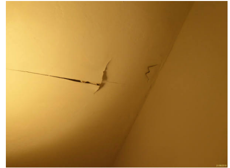
Ceiling paintwork perishing
