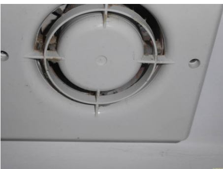
Vent casing dusty
