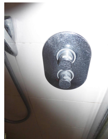
Shower controls limescale marked
