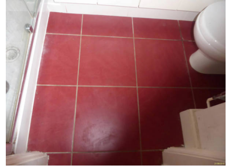
Flooring not clean
