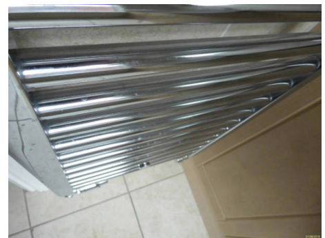
Stains/marks on ladder radiator
