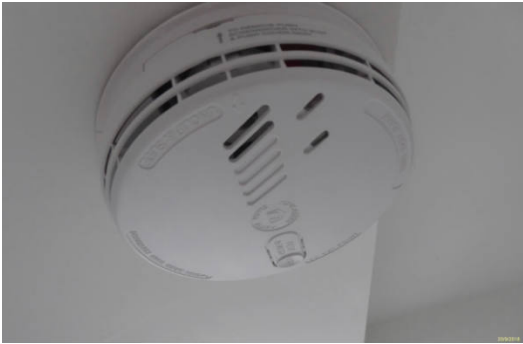
Smoke alarm - Top landing
