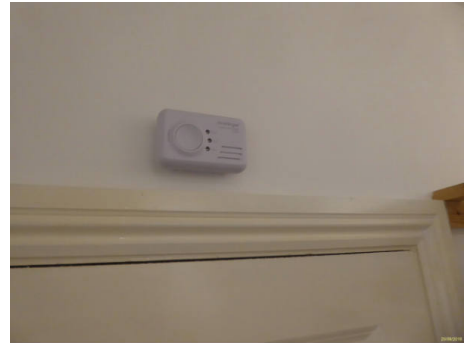
CO alarm - utility
