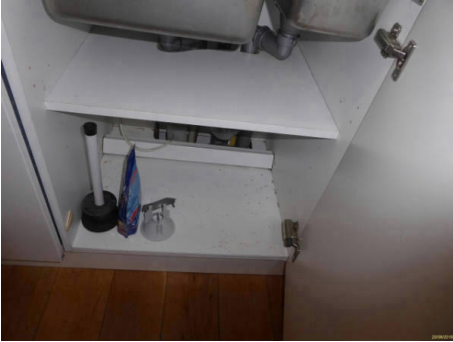
Under sink unit
