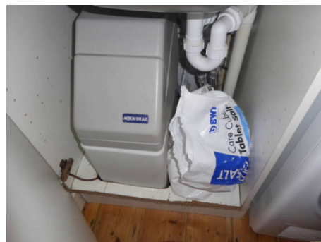
Under sink unit
