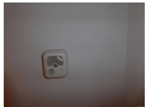
Smoke alarm - mid landing
