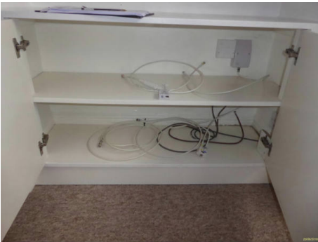
Cupboard with misc cabling
