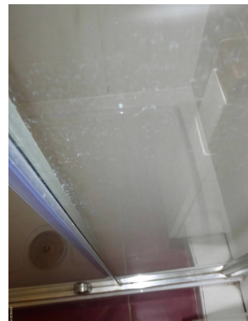
Limescale shower glass panels
