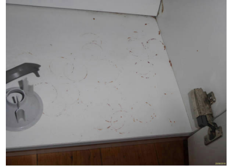
Ingrained marks under sink unit
